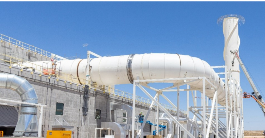
New infrastructure on the surface supports airflow underground [public domain, U.S. DOE.]
