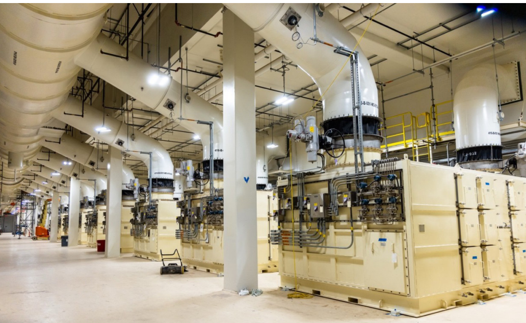
Interior of the New Filter Building at WIPP, showing completed HEPA filter arrays and airflow control systems powering the Safety Significant Confinement Ventilation System (SSCVS) [Public domain, U.S. DOE]
