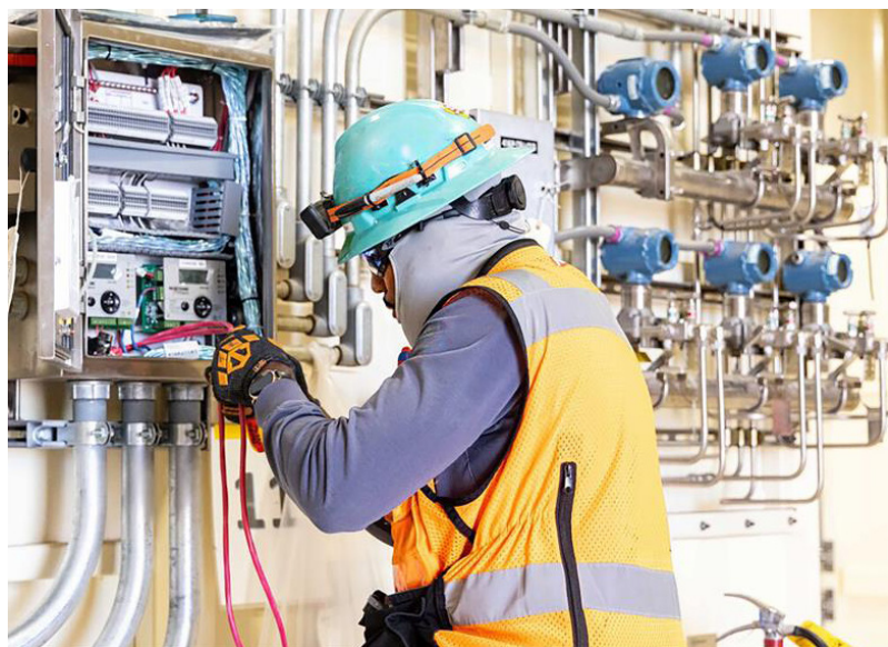
A control panel undergoes testing at the newly constructed Safety Significant Confinement Ventilation System [public domain, U.S. DOE]
